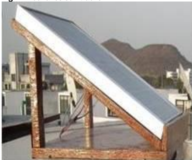
Fig.3 Tilted fixed PV panel
