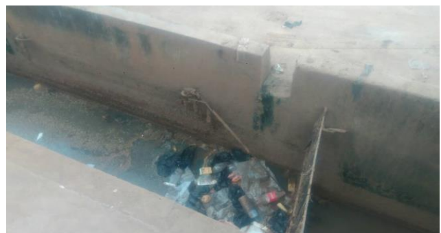
Plate 6: Drainage dumping attitude
